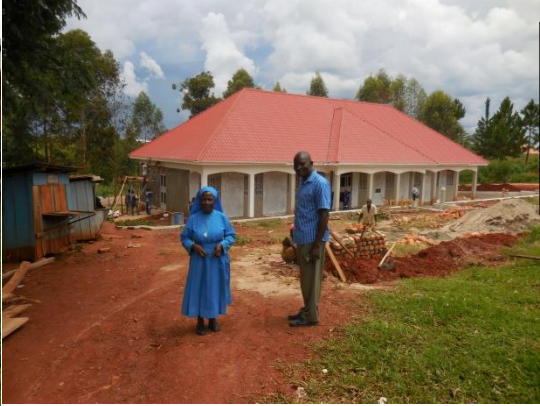
St Luke Health Center new out-patient building. Sr Maria Goretti and Cyprian in charge of the expansion
